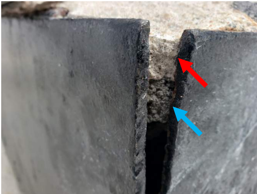
Figure 18. Edge of dome cap concrete slab. A layer of white material (red arrow) was noted on top of a layer of gray material (blue arrow).
